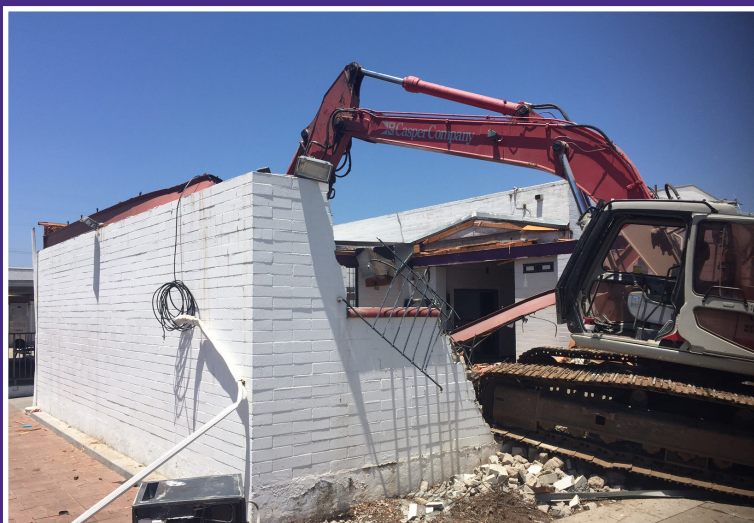
There goes the weight room wall.
