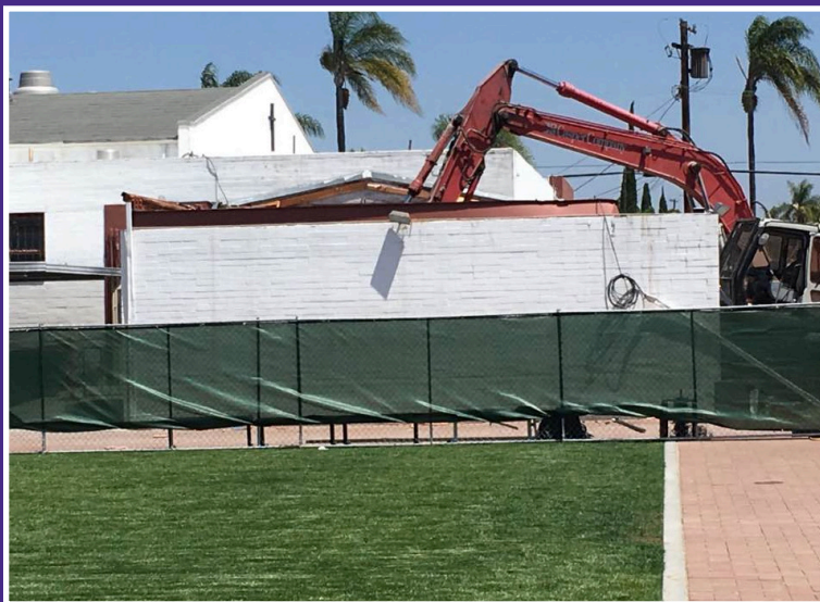
Construction began this summer on the transformation of old Dougherty Gym into a multi-purpose drama and arts center.
